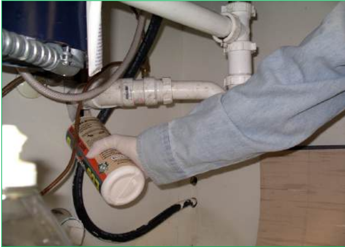
Figure 11. Applying dust to a wall void where plumbing pipes enter the wall.
