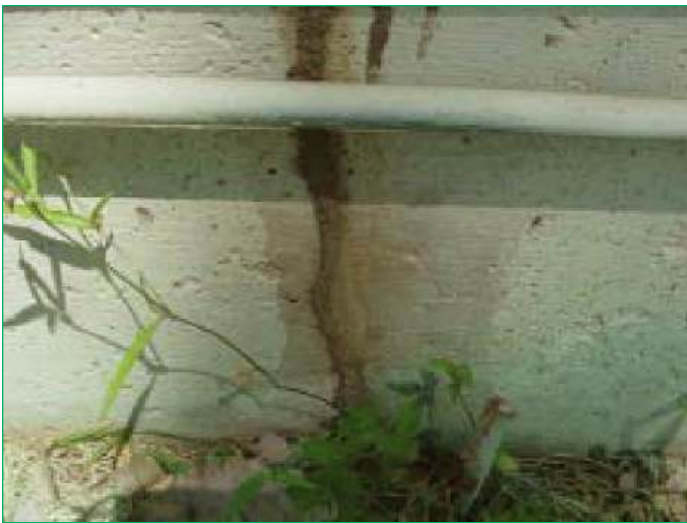
Figure 11. Shelter tube of an active termite colony.
