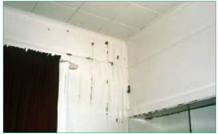
Figure 12. Shelter tubes on interior walls.
