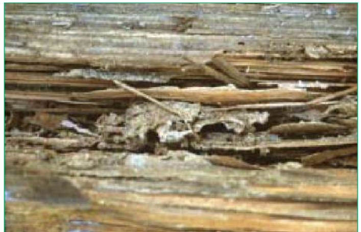
Figure 10. Formosan subterranean termite damage to early- and late-season wood.
