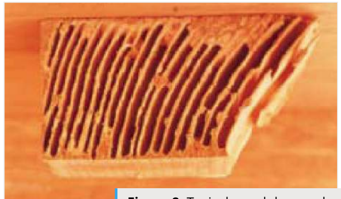
Figure 8. Typical wood damage by subterranean termites.
