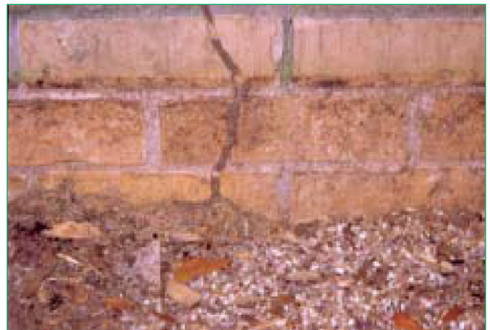
Figure 6. Subterranean termite shelter tubes on foundation wall.
