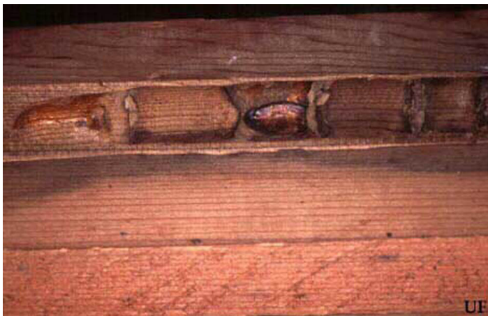
Figure 7. Internal damage to structural wood by a large carpenter bee, Xylocopa sp., showing individual larval cells. Credits: University of Florida
