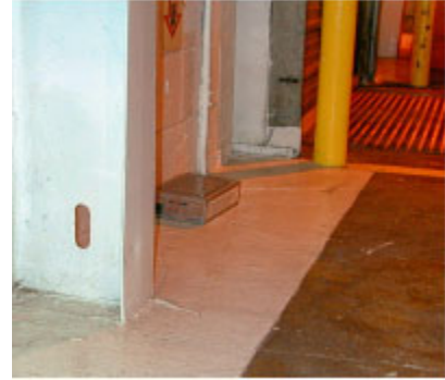
Figure 2. Interior mouse traps along a food distribution wall. Such traps are an important component of proactive rodent control programs. But they are not more important than proactive inspections for rodent activity away from wall areas.
