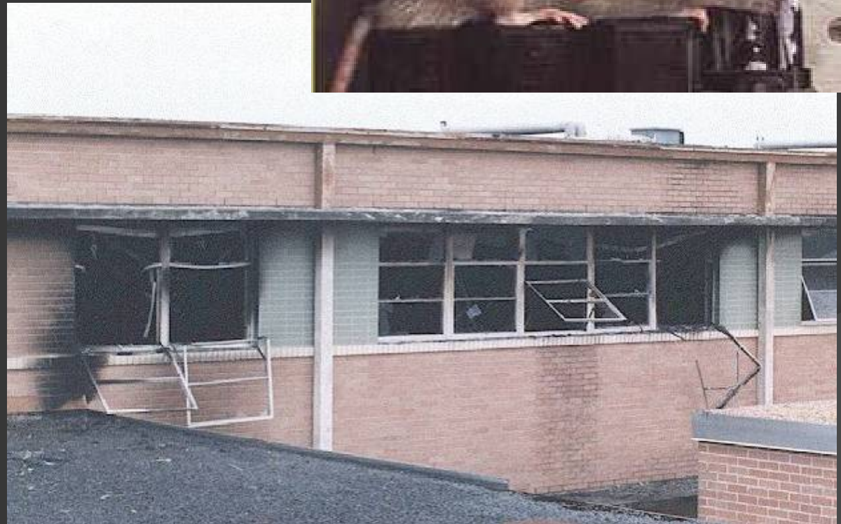
School building destroyed by fire
