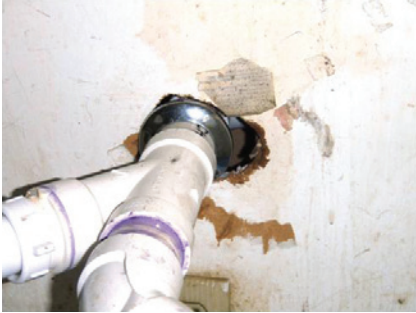
FIGURE 2 • An improperly installed escutcheon plate can be repaired by the college/university maintenance section.
