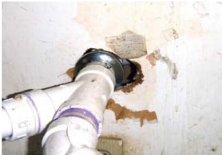
Figure 2. An improperly installed escutcheon plate can be repaired by the DOHRE Maintenance Section.
