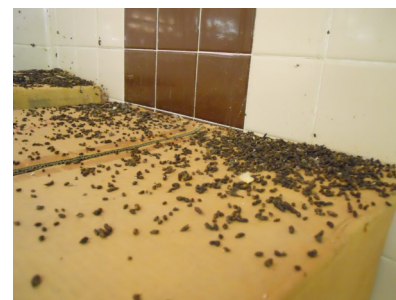
This kitchen storage room had bats living in the false ceiling area. In the top image is evidence of staining, while the bottom image is evidence of bat guano.
