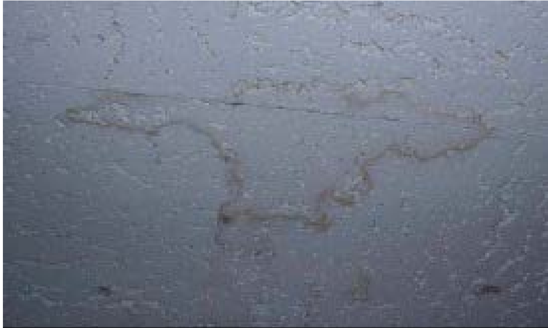
Rodent urine stain in drop ceiling
